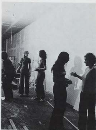
1972: Founding members renovating space at 97 Wooster Street prior to opening of gallery.
