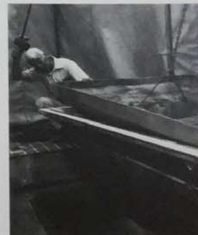
(Top) FRC panels are made by spraying a concrete slurry and chopped glass fibers into an architectural form.
