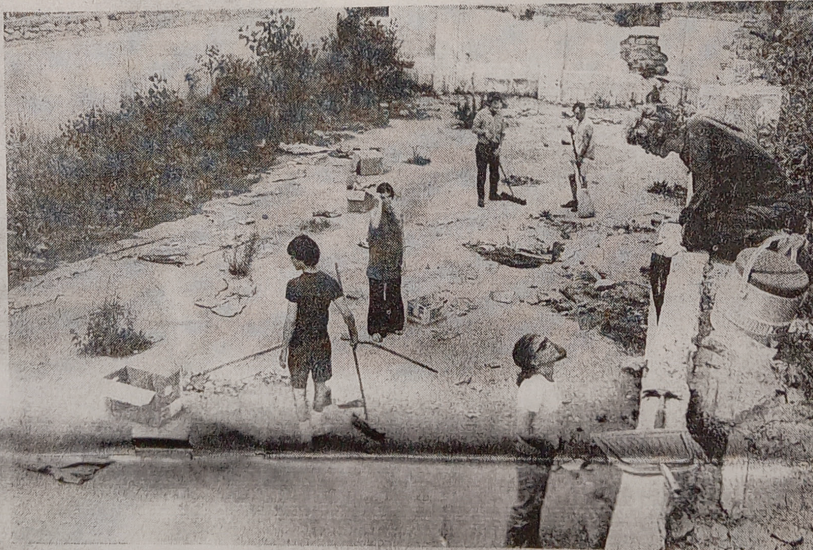
ON BECOMING—The site of an empty hole at Washington and Linn Streets is becoming a work of art. University of Iowa students who are cleaning up the hole, where a furniture store once stood, say their cooperative acts and the improved site constitute the work of art. They
