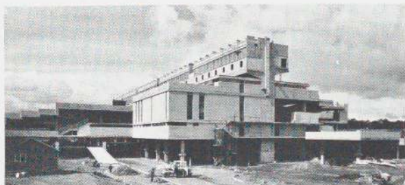
Cumbernauld's town center, in construction, runs along the ridge and encases the spinal highway. Geoffrey Coppitt, architect in charge.
